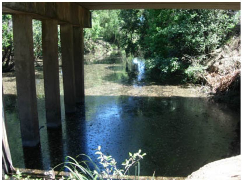
Looking downstream under D'Aguilar Highway bridge over the Stanley River, half a kilometre west of Woodford, on the way to Kilcoy. One hundred metres upstream a large log blocks the river.
